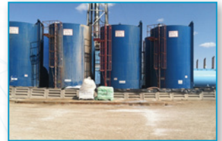
Fuel Tank Monitoring
